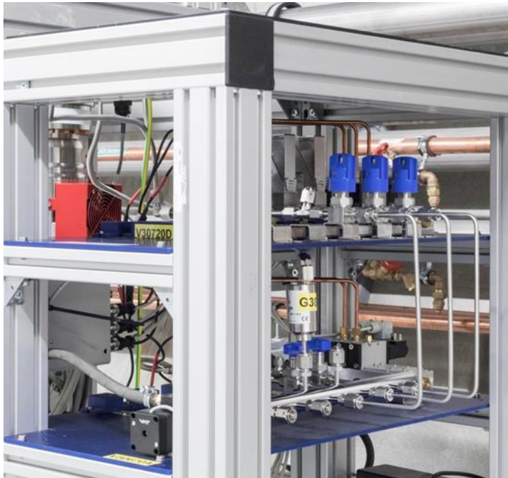
Figure 10: Detail view of the CGI high purity gas manifold
