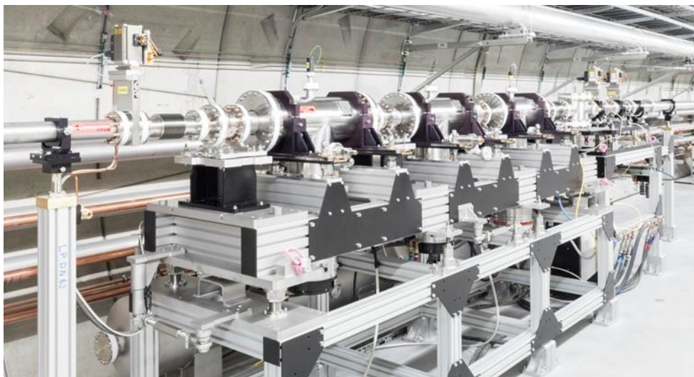
Figure 14: Current tunnel installation of the gas attenuator upstream differential system
