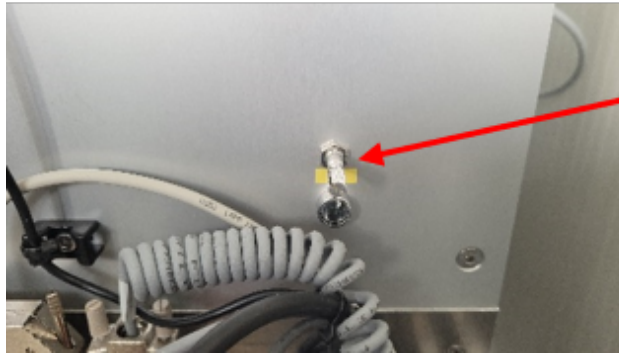
Switch and potentiometer for Leak rate sound
